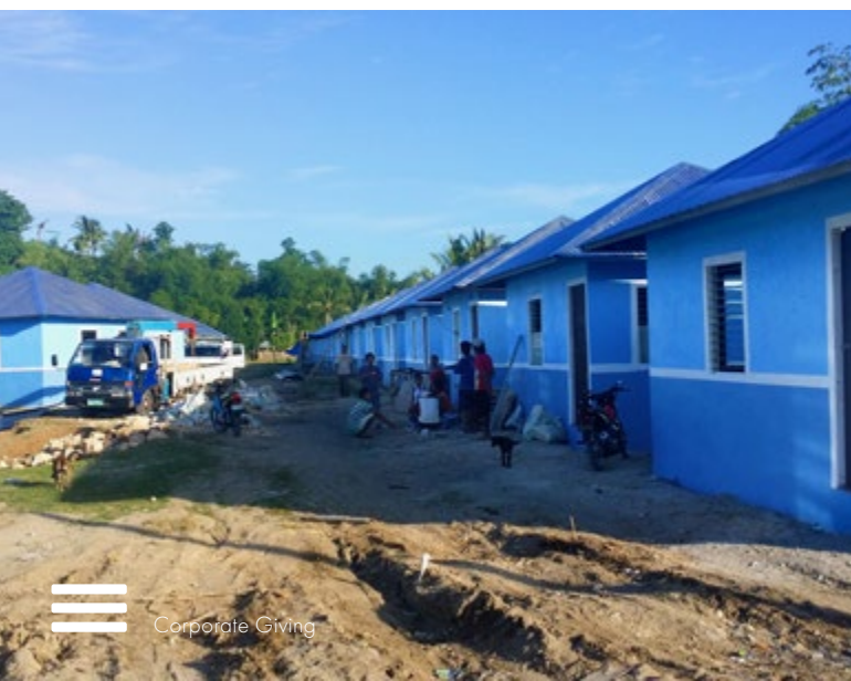
Habitat for Humanity Philippines developing new homes in Barangay Margen in Ormoc, Leyte.
